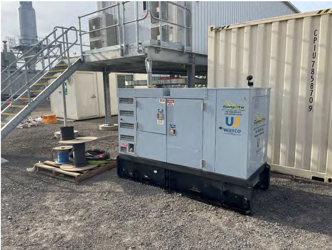
Compressor station – self-bundled diesel generator
