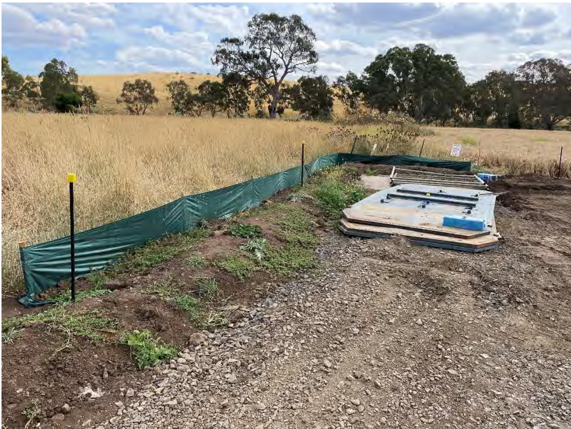
KP16.8 HDD at Deep Creek – earthen bunding and sediment fencing on the downslope part of site
