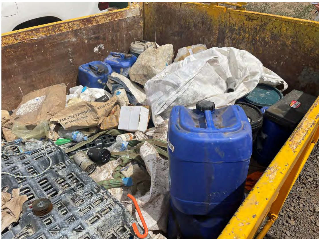
KP3.3 HDD at Melton Highway – example of poor storage of waste
