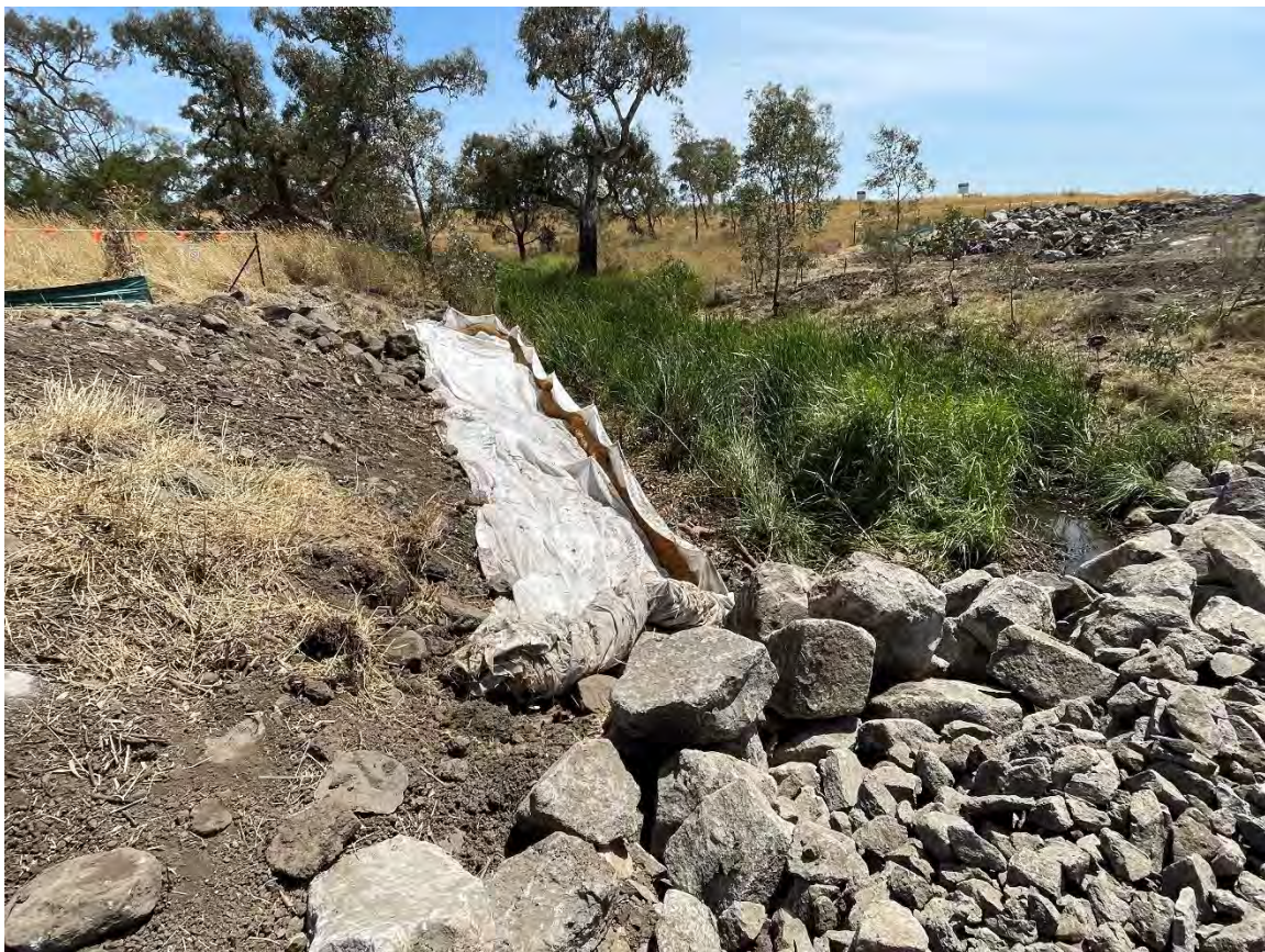
KP42 Merri Creek – view across creek bank showing erosion and sediment controls
