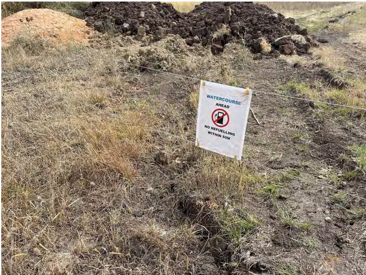
KP10.5 Unnamed tributary of Jackson's Creek – refuelling signage
