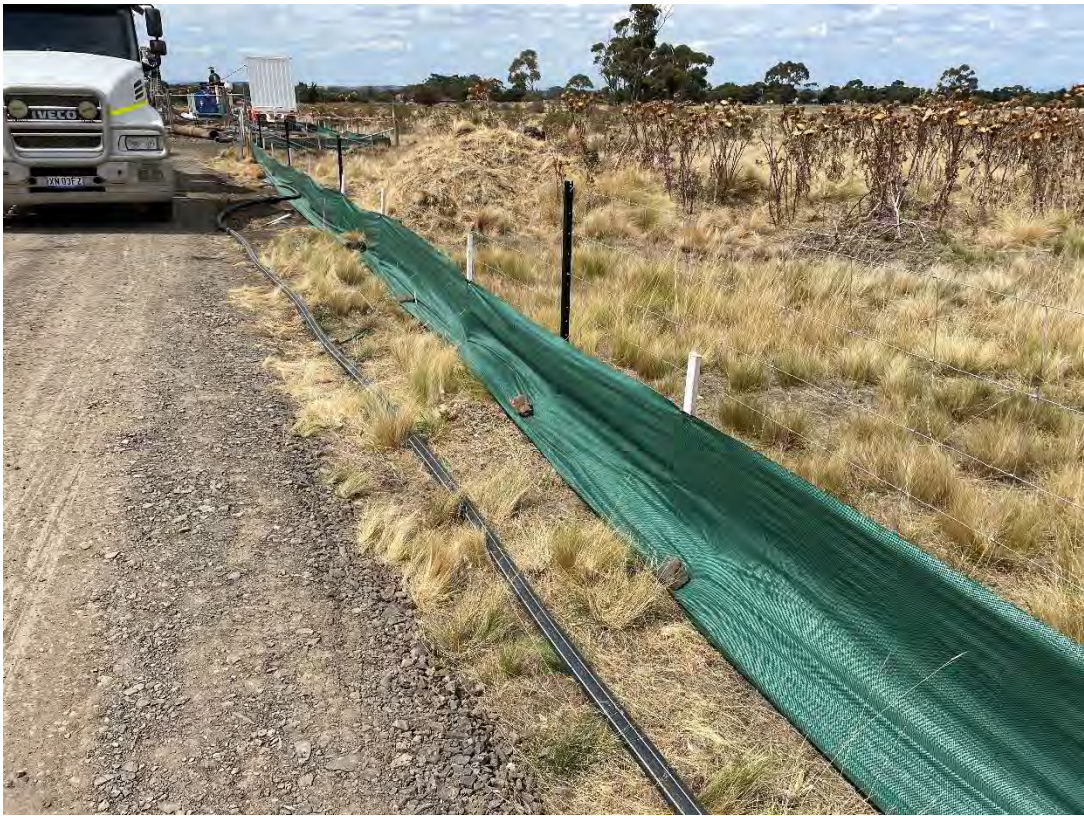
KP8.8 HDD at Calder Highway – entrance to HDD site showing poor installation of sediment fencing
