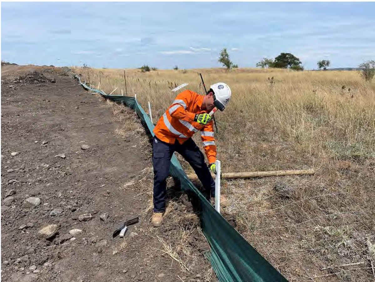
KP43 – repairs to sediment fencing by Spiecapag Environment Advisor
