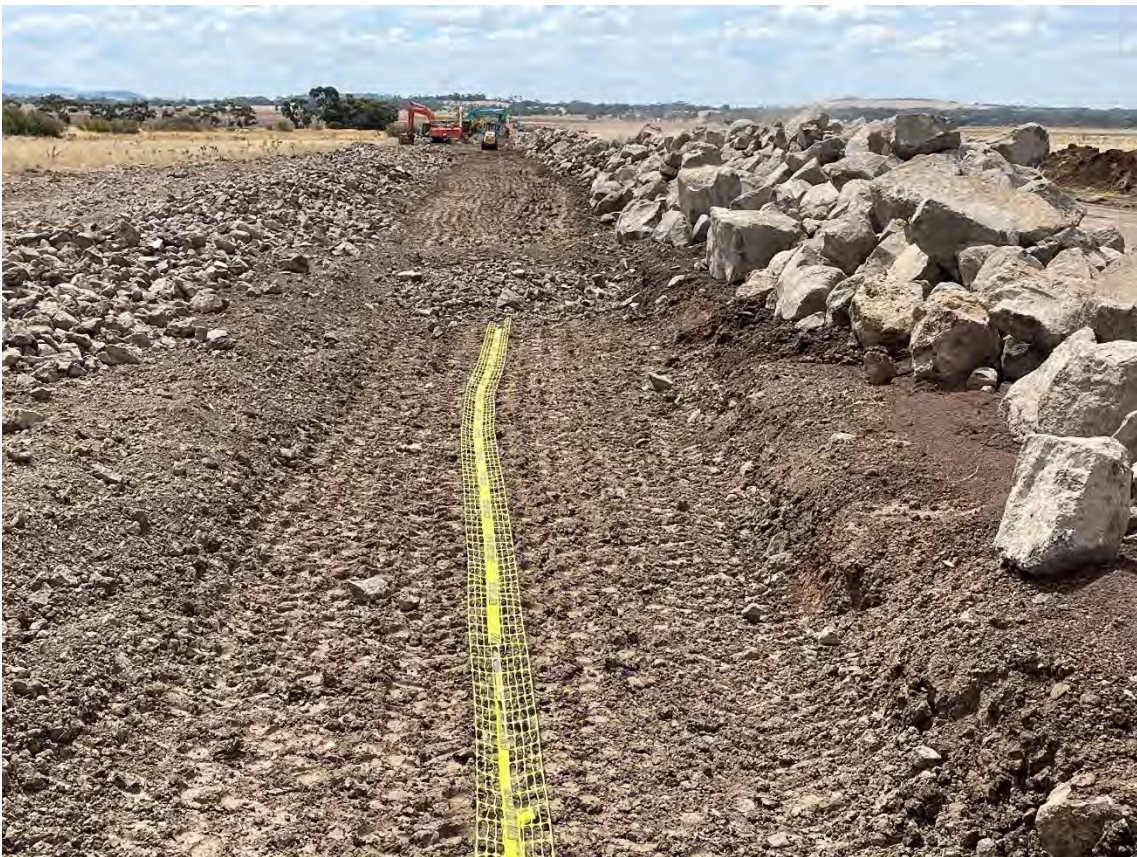
KP5 – reinstated trench spoil showing hazard taping prior to topsoil reinstatement
