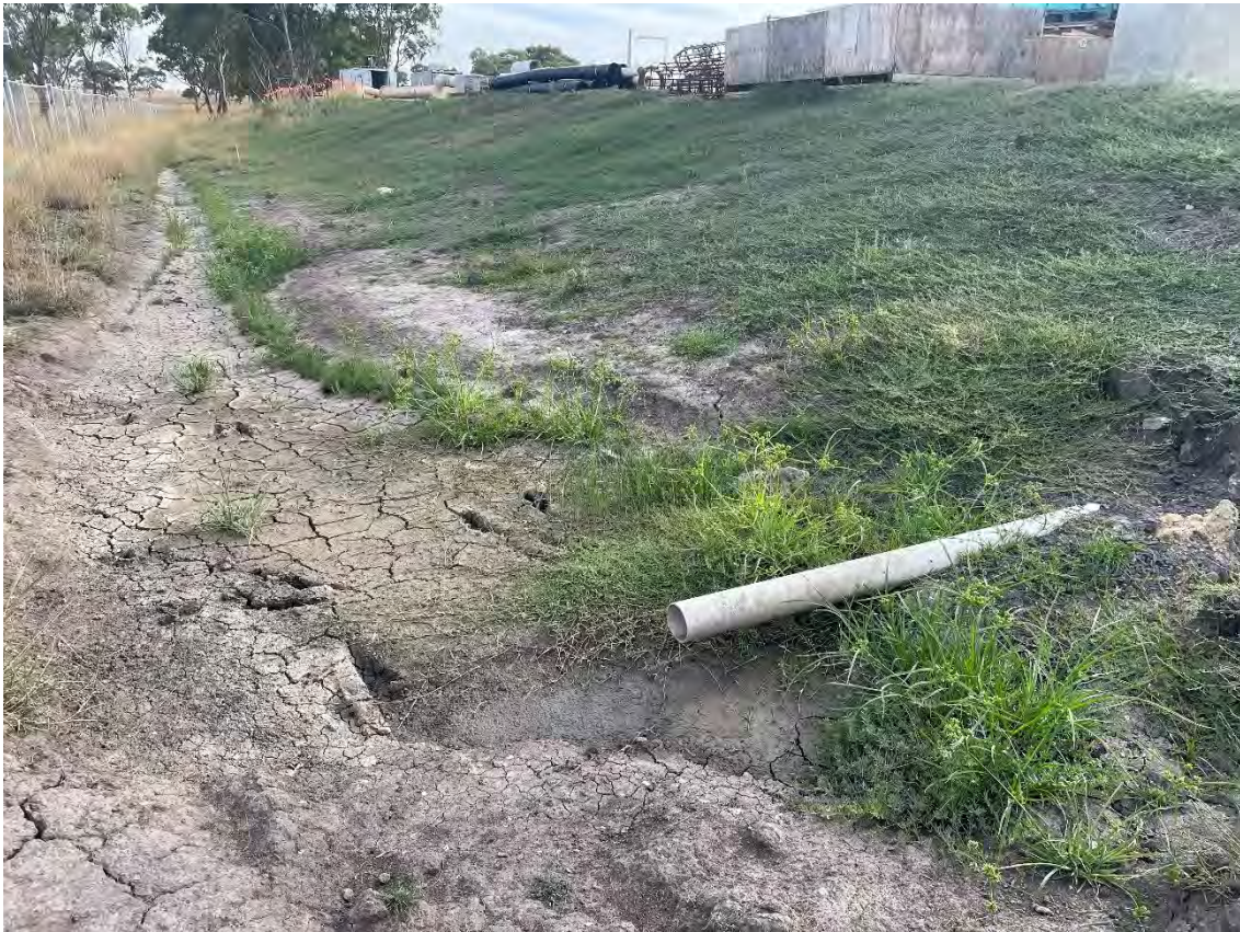
Compressor station – bottom of batter, with minimal scouring and good vegetation cover
