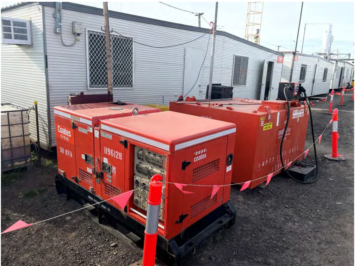
Compressor station – diesel storage with bowser, pump and drip tray
