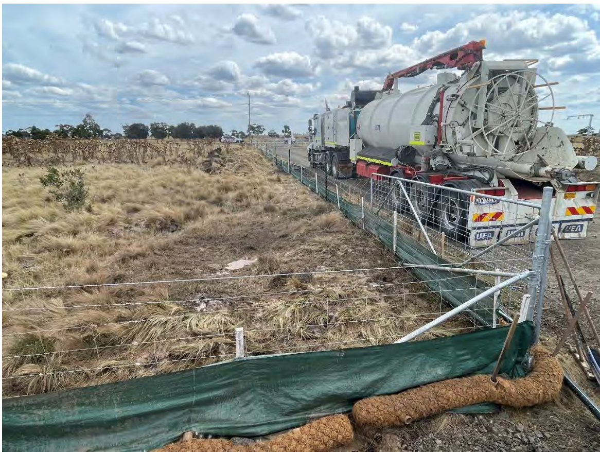
KP8.8 HDD at Calder Highway – minor frac-out beyond the site perimeter
