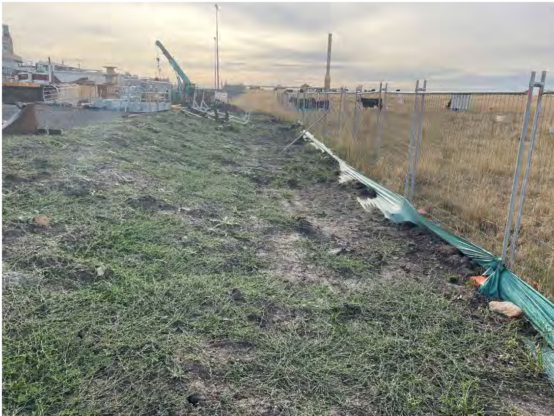
Compressor station – sediment fencing downslope of the batter, preventing movement of soil off site
