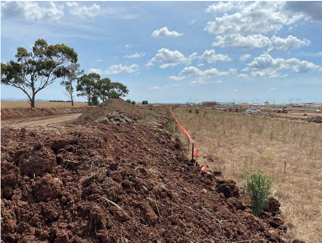
KPO Fraser Rise – minor excursion of topsoil beyond the flagged construction RoW
