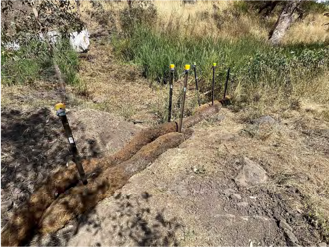
KP42 Merri Creek – coir logs that need to be properly installed to control runoff
