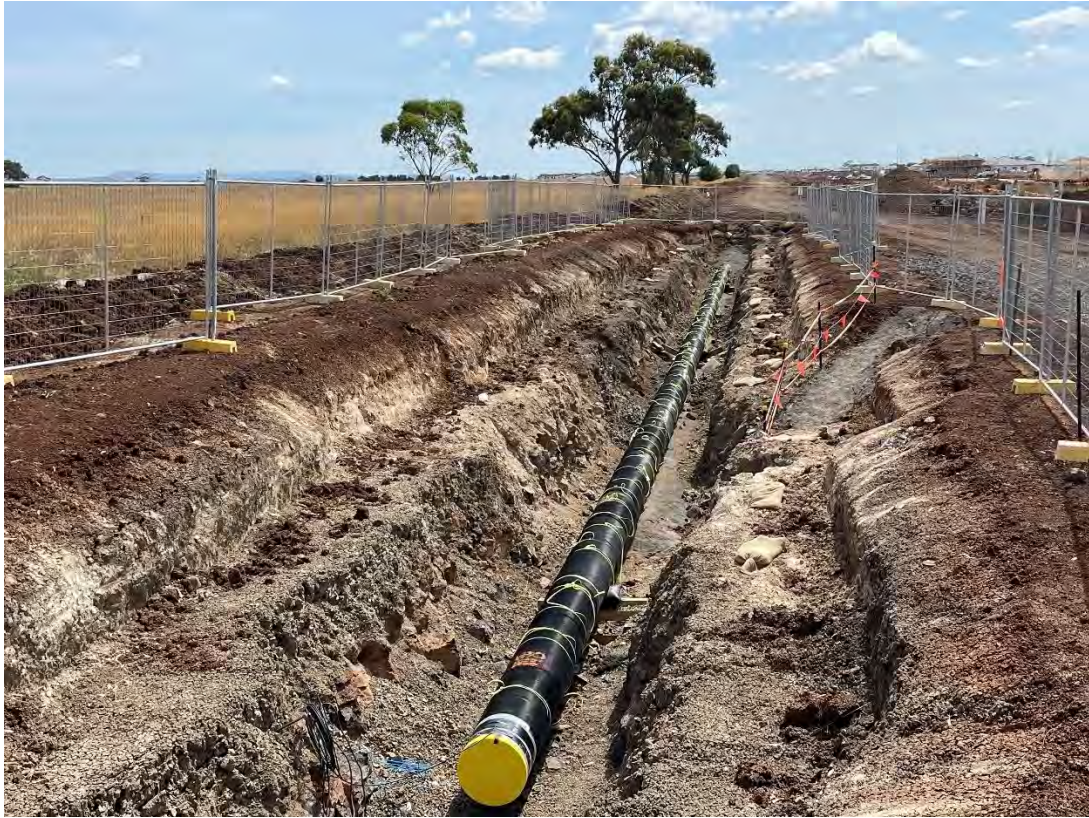
KPO Fraser Rise – benched open trench, fauna caps on pipe, fenced to prevent fauna ingress
