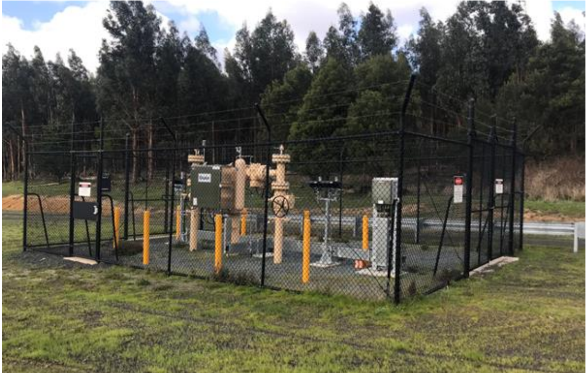
Figure 2 Typical mainline valve facility
