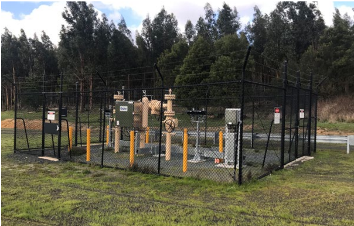
Figure 4-6 Typical mainline valve facility
