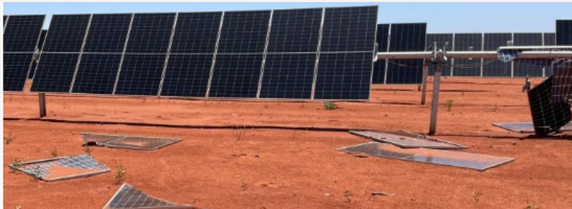
Gruyere Solar Farm following storm event
