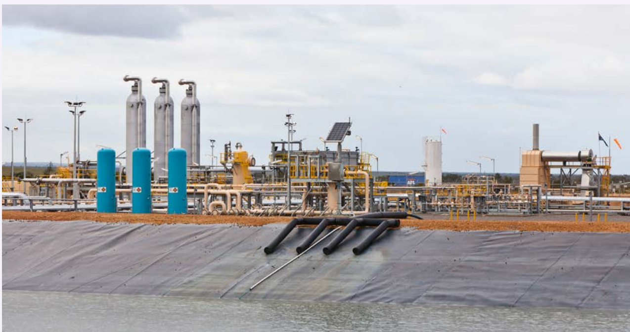
Mondarra Gas Storage Facility, Western Australia
