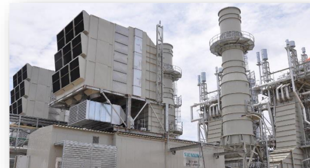
Diamantina Power Station in Queensland
