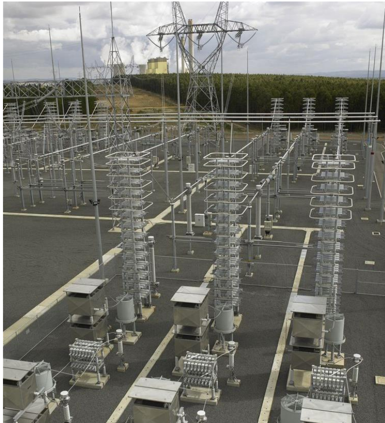
Triple tuned harmonic filter in Loy Yang AC yard
